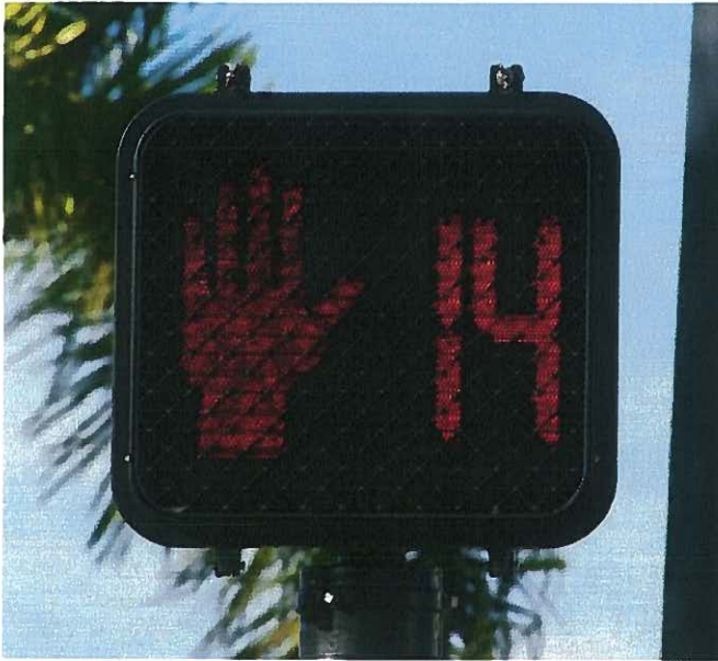
Figure 3 – Countdown Pedestrian Signals
