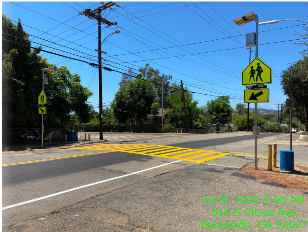
Figure 5: Solar Powered RRFB, signage and high visibility crosswalk in place.
