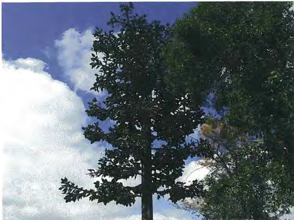
Figure 6: Cricket Communications Antennas #26 through #28
