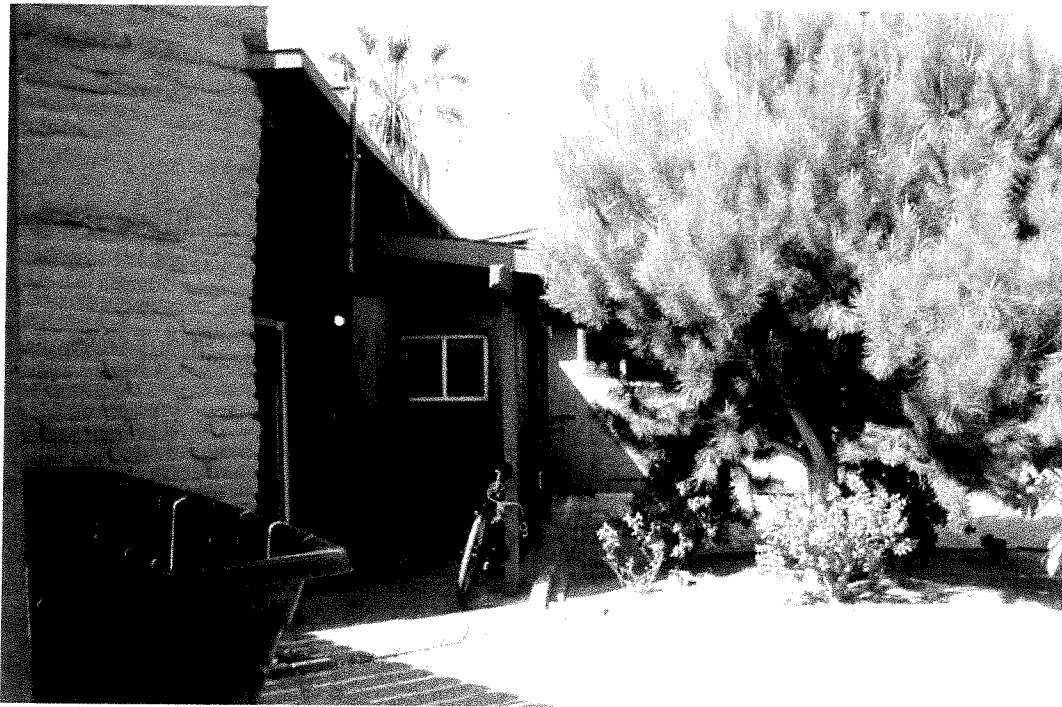
Image 11: Looking west from the inner court at portions of the east façade and porch. Note the windows have been replaced with vinyl sliders.
