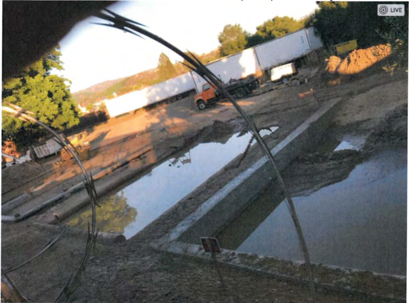
7/18/2019 - PHOTO OF SOUTH PITS; NO EARTHEN BERM RETENTION POND TO SOUTH OF PITS BEHIND TRUCK IN PHOTO (SEE 8/11 PHOTO)
