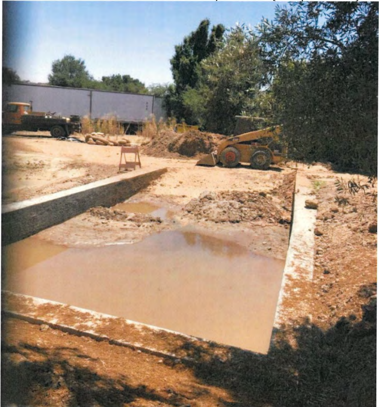
7/18/2019 - PHOTO OF SOUTH FAR WEST PIT; NO EARTHEN BERM RETENTION POND TO THE SOUTH BY TRUCK/DIRT PILE (SEE 8/11 PHOTO)
